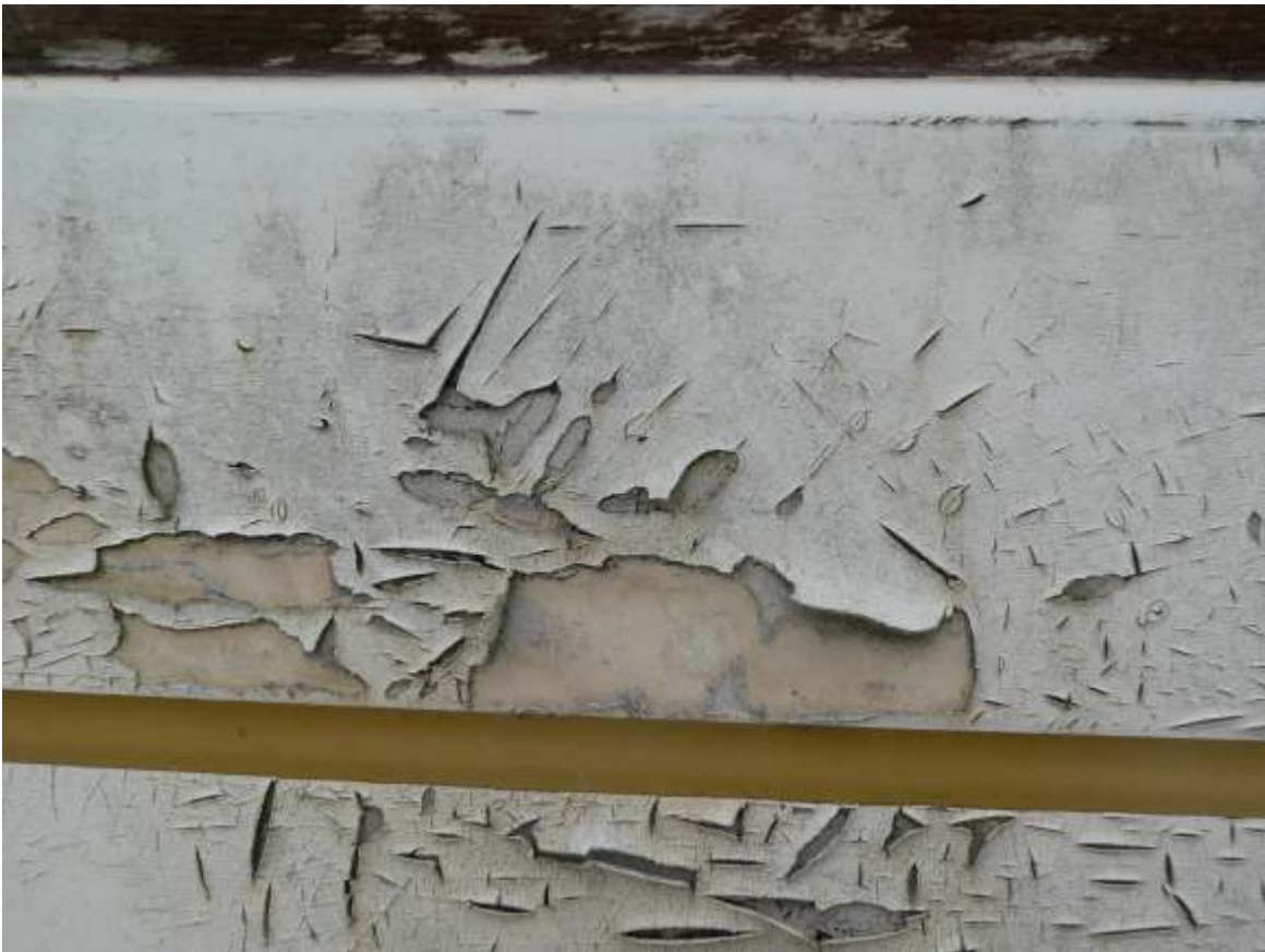
Details of paint damage to the hull side. Paint will have to be sand away down to fiberglass and redone from scratch, note that the fiberglass itself is not damage.
